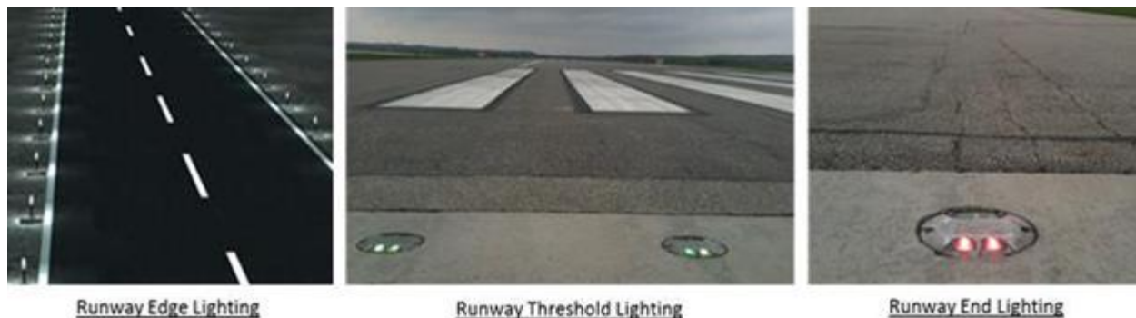
Figure 4.13. (Added-WRIGHTPATTERSONAFB) Typical Runway Lighting.
