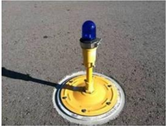
Figure A3.15. (WHITEMANAFB) Taxiway Edge Light.
