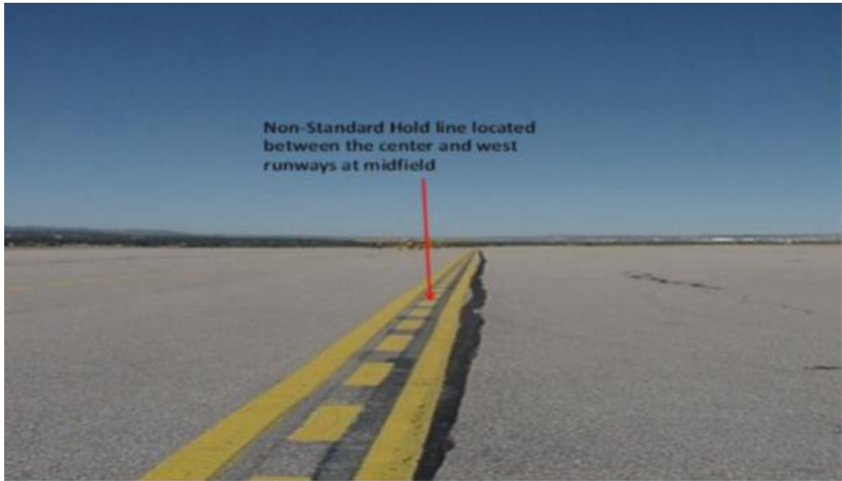
Figure A11.3. (Added-USAFA) Non-Standard Hold Line Marking Between Center & West Runways.
