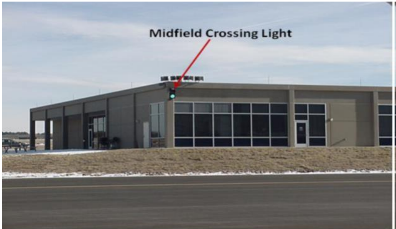
Figure A11.15. (Added-USAFA) Taxiway Crossing Light.
