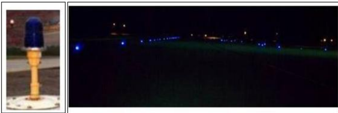
Figure 4.11. (Added) Taxiway Lights.
