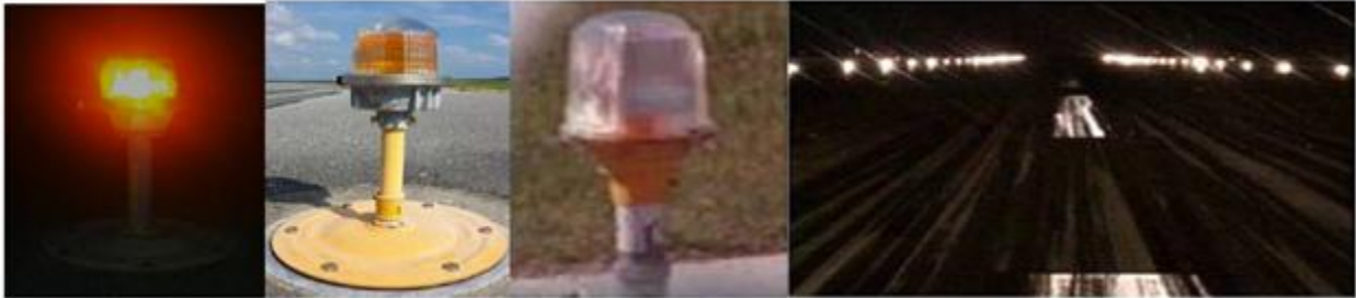
Figure 4.10. (Added) Runway Lights.
