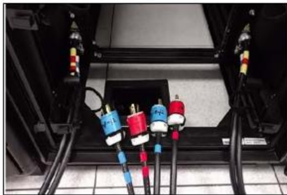
Figure A3.1. Example Power Strip Markings 1.
