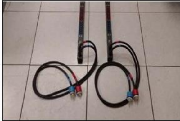
Figure A3.2. Example Power Strip Markings 2.
