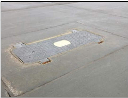
Figure 4.9. (Added) In-Ground Fuel Pit (Echo Row).
