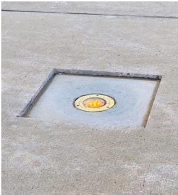
Figure A3.4. (MALMSTROMAFB) Airfield Lighting.
