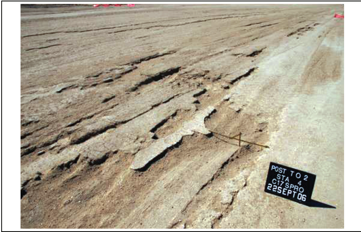
Figure 9.3 Jet Blast Erosion
