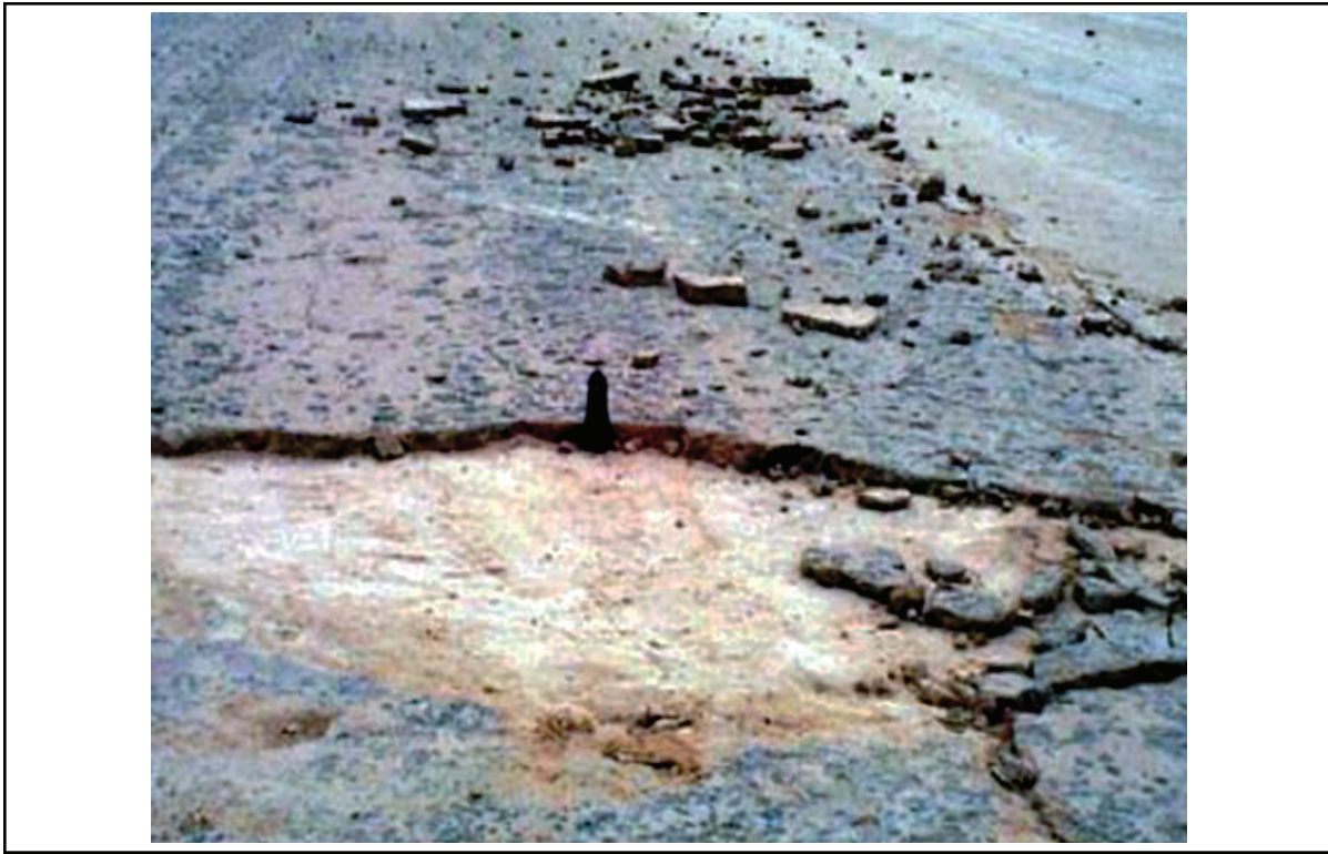
Figure 9.4 Stabilized Layer Failure
