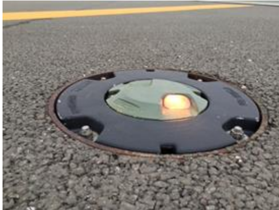
Figure A3.13. (Added-LAKENHEATHSUP) Taxiway Edge Light.
