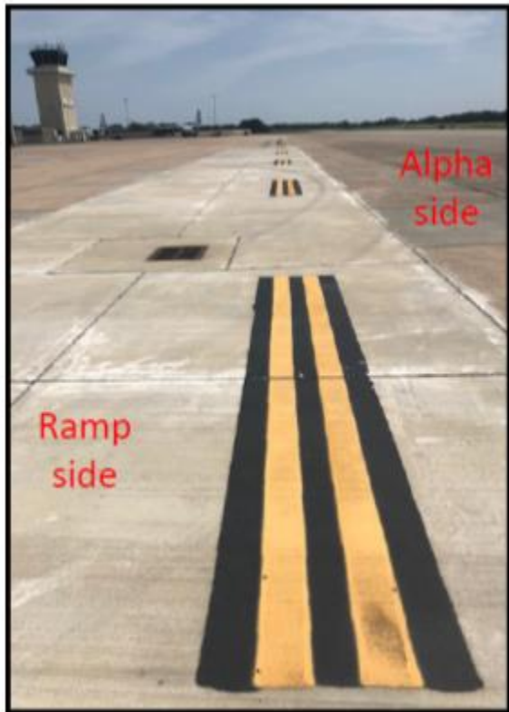
Figure 4.2. (Added-KEESLERAFB) Taxilane Edge/Wingtip Clearance Markings.
