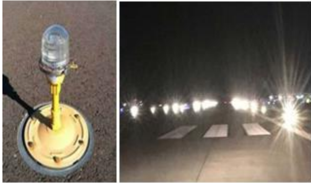
Figure A11.6. Edge Runway Lights.
