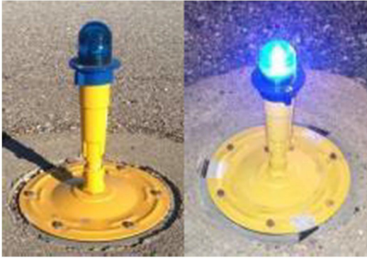
Figure 4.9. (Added) Taxiway Edge Light.
