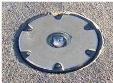
Figure 6.16. Taxiway Edge Light.
