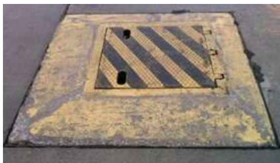
Figure 5.4. Centralized Aircraft Support System (CASS) Pit.
