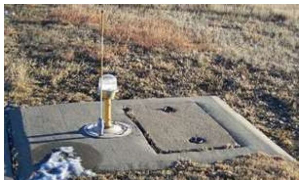
Figure 6.15. Runway Edge Light.
