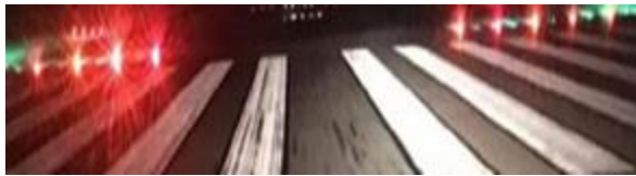
Figure 4.36. (Added-EDWARDSAFB) .Combined Runway Threshold and Runway End Light.
