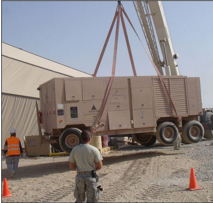
Figure 1.4. Prime Power Generators Support Sustained Operations
