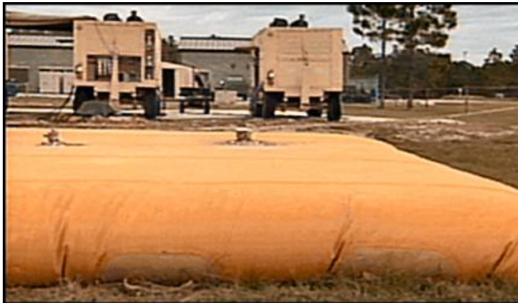
Figure 7.7. Generators with 10,000-Gallon Fuel Storage Bladder
