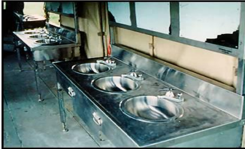
Figure 10.14. Shave Facility Washstand
