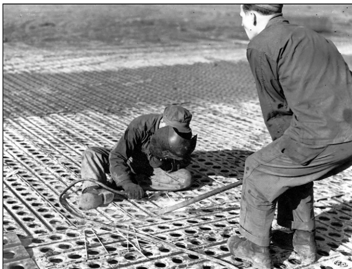
Figure A4.15. Damaged PSP Being Repaired.
