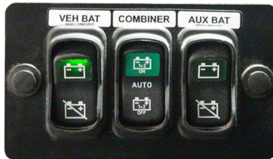
Figure 3.2 Battery disconnect switch
