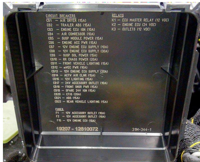
Figure 5.2 mVEC with faulted breakers
