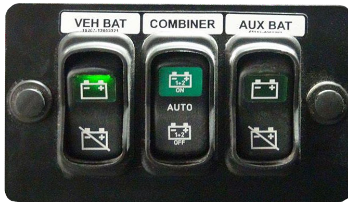
Figure 2.24 Battery disconnect switch panel
