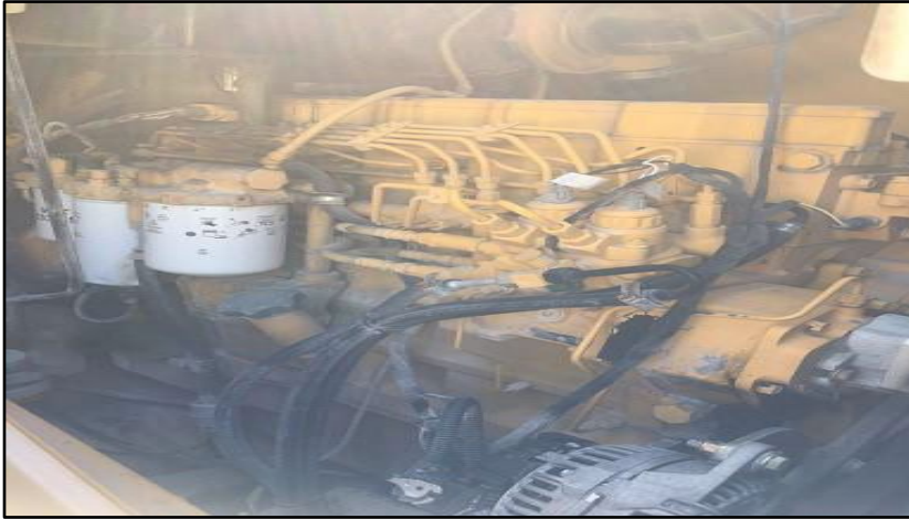
Figure 5.1. Engine Oil check.
