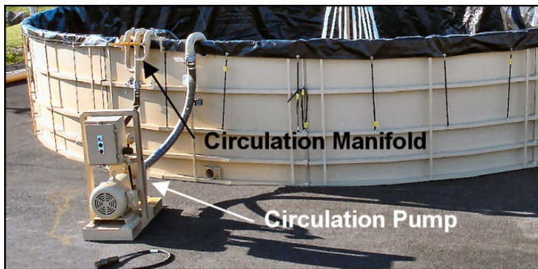
Figure 5.21. Circulation Pump Positioned Below Circulation Manifold.
