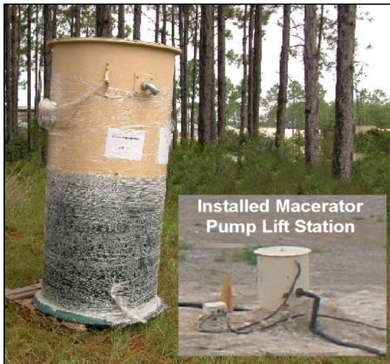
Figure 5.15. Macerator Pump Lift Station.
