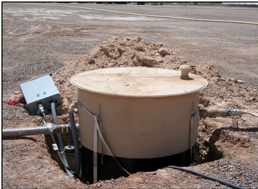
Figure 5.16. Dual Pump Lift Station.
