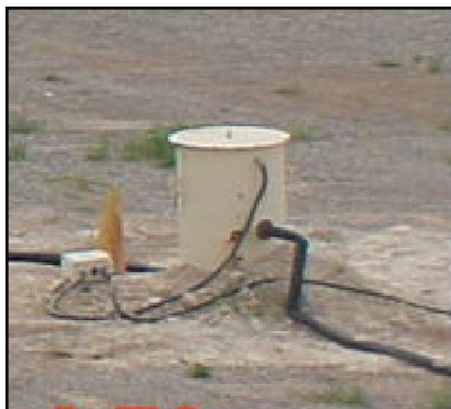
Figure 6.19. Installed Macerator Pump Lift Station.
