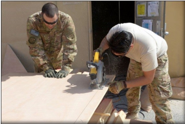
Figure 1.5. Prime BEEF Building Army Tactical Operations Center.
