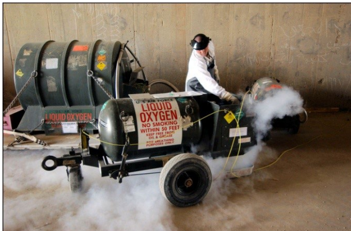
Figure 3.6. Liquid Oxygen Storage and Servicing Facility.
