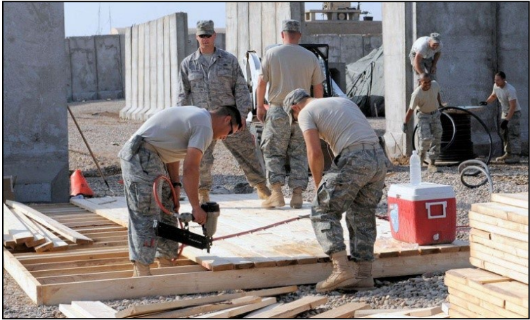
Figure 5.2. Building Shower Facilities at Contingency Location.
