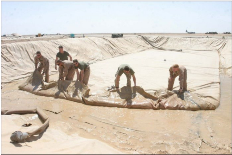
Figure 4.11. Fuel Dikes Control Spills and Forms Protective Barrier.
