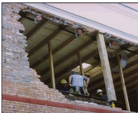
Figure 4.34. Damaged Brick Infill Wall.
