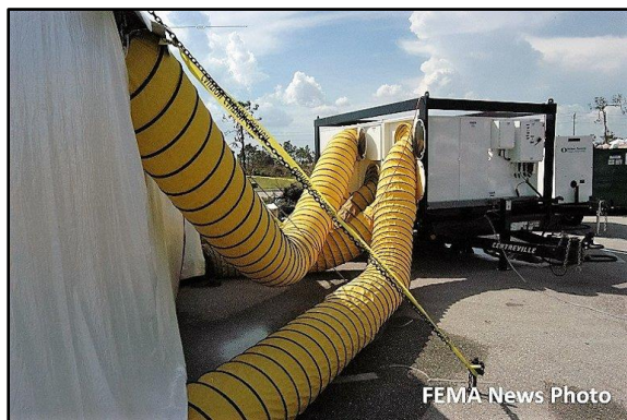
Figure 8.5. Trailer-Mounted Portable AC Unit.
