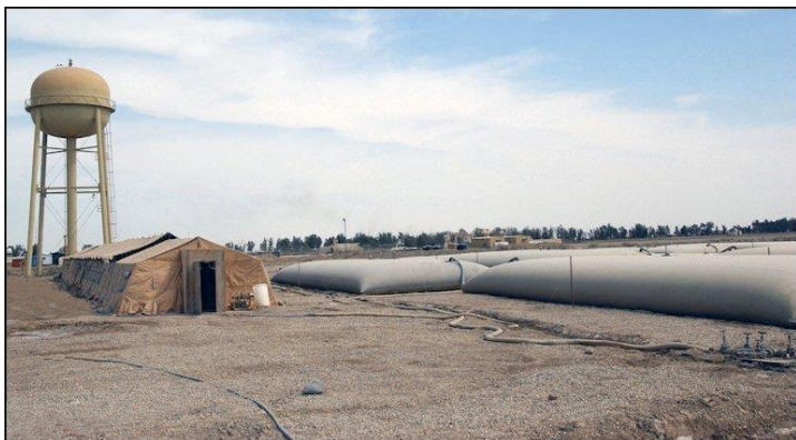
Figure 5.15. Temporary Water Storage Bladders.
