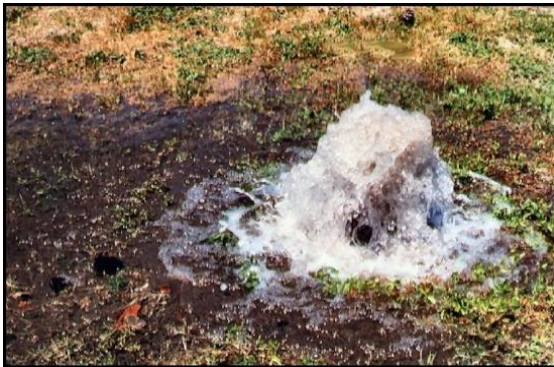
Figure 5.2. Obvious Water Line Break.
