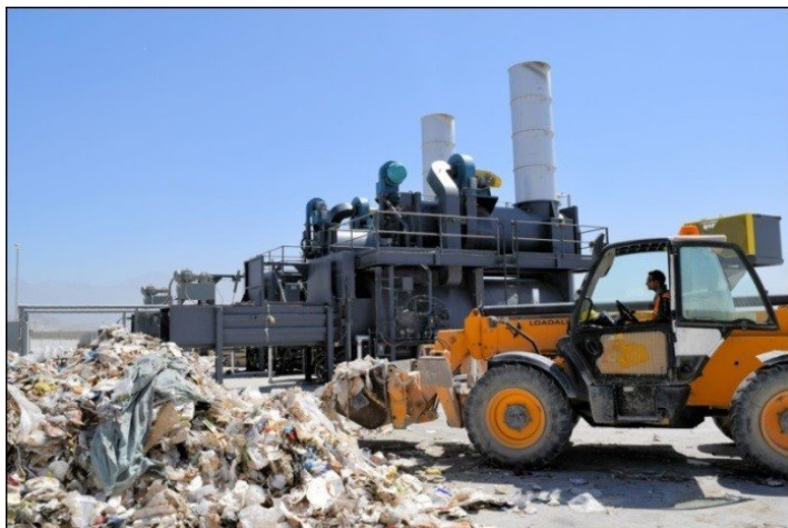
Figure 5.5. Solid Waste Incinerator Complex at Bagram Air Field.
