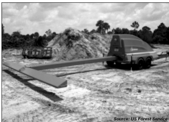
Figure 5.9. Trench Burner ACD.
