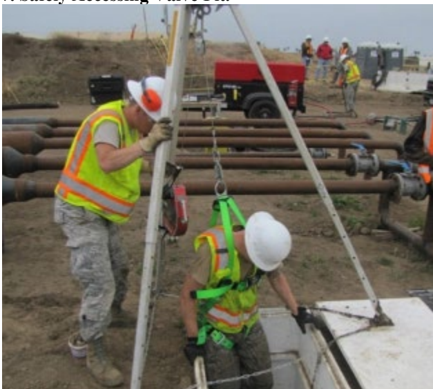
Figure 3.27. Safely Accessing Valve Pit.
