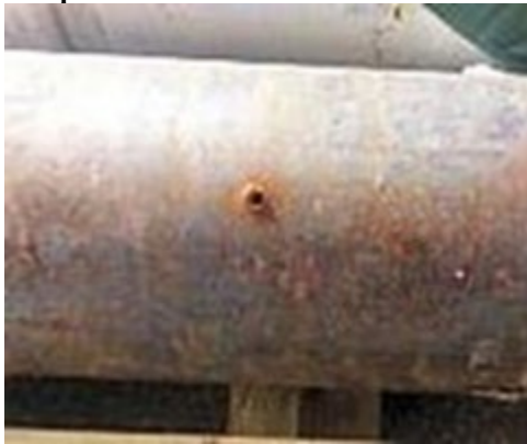
Figure 3.1. Hole in Pipe Wall.
