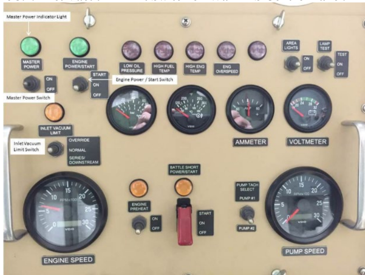
Figure 5.7. Inlet Vacuum Limit Switch on WaFERS Control Panel.
