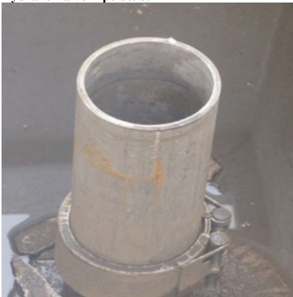
Figure 3.29. Hydrant Valve Pipe Stub.
