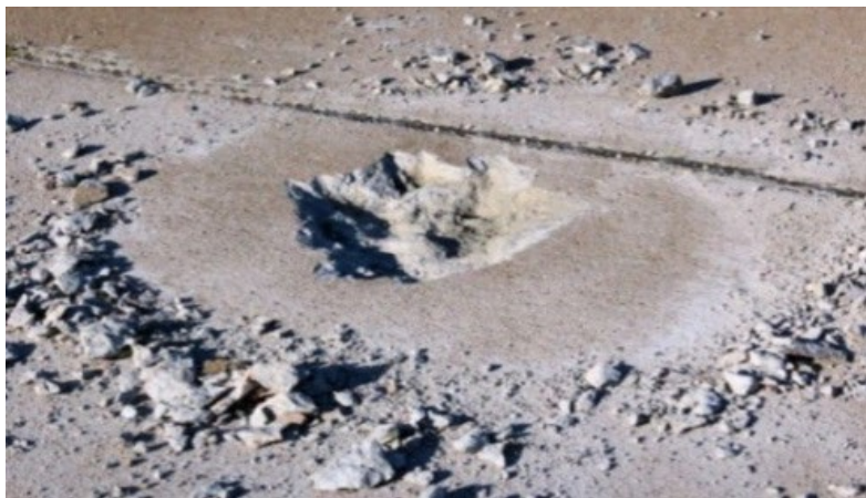
Figure 8.8. Spall Prepared for Expeditious Repair.
