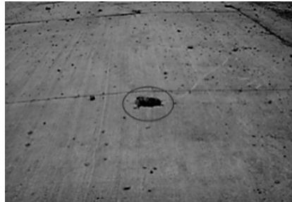
Figure 3.6. Camouflet in Concrete Surface.
