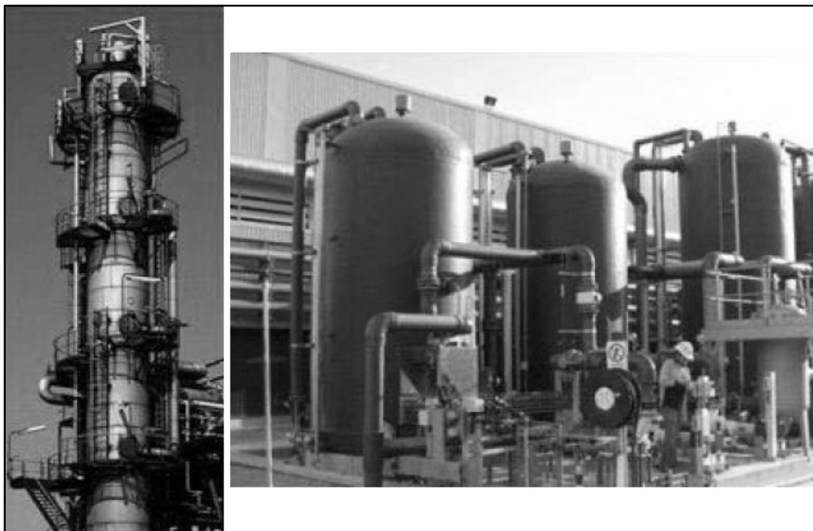
Figure G-3. Example chemical storage tanks and distillation tower
