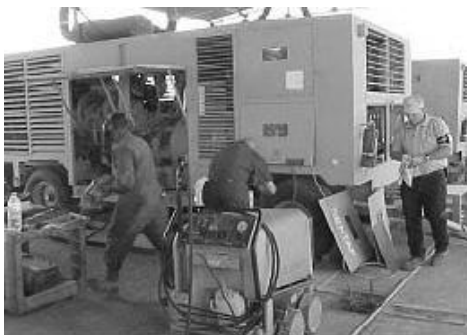
Figure 2.2. Providing Electrical Support at Deployed Location.
