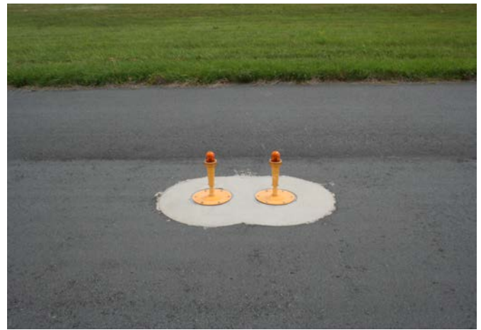
Taxiway End Lights
