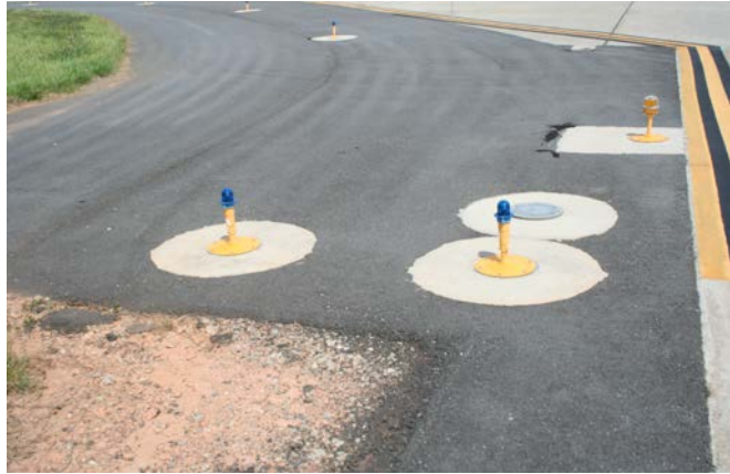
Taxiway Edge Lights
