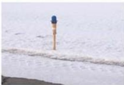
Figure 4.16. (Added-3WG) Taxiway Lights.
