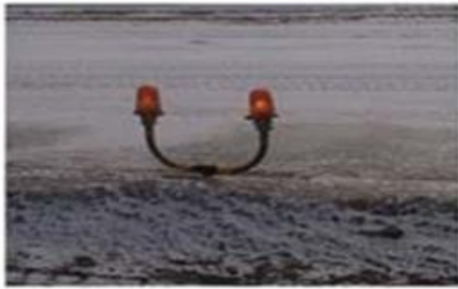
Figure 4.17. (Added-3WG) Taxiway End Lights.
