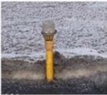
Figure 4.15. (Added-3WG) Runway Edge Lights.
