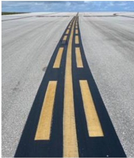
Figure 4.7. Example of an Enhanced Taxiway Centerline.
