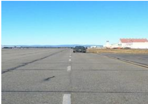
Figure 3.9. Vehicle Lane Marking.
