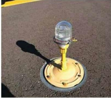
Figure A10.9. Runway Edge Light
