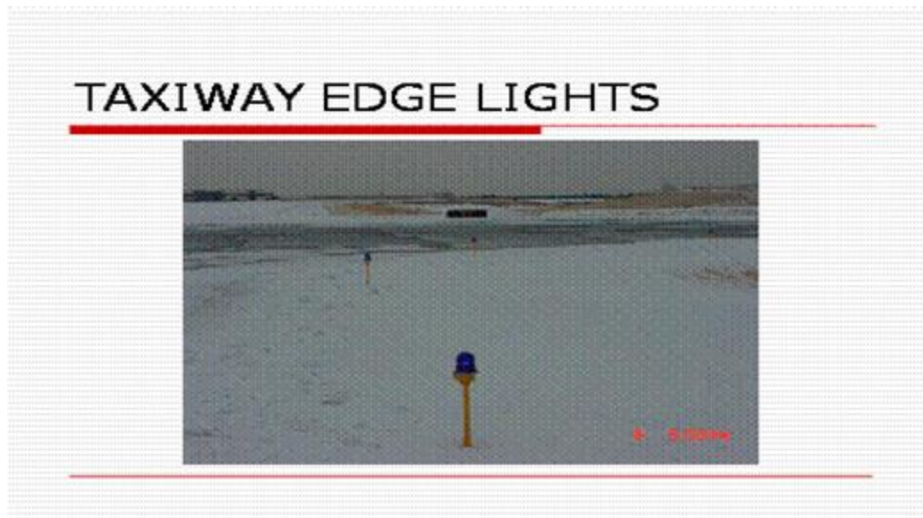
Figure A5.2. Taxiway Lights.
