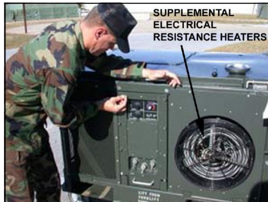
Figure 4.7. Supplemental Electric Resistance Heaters.
