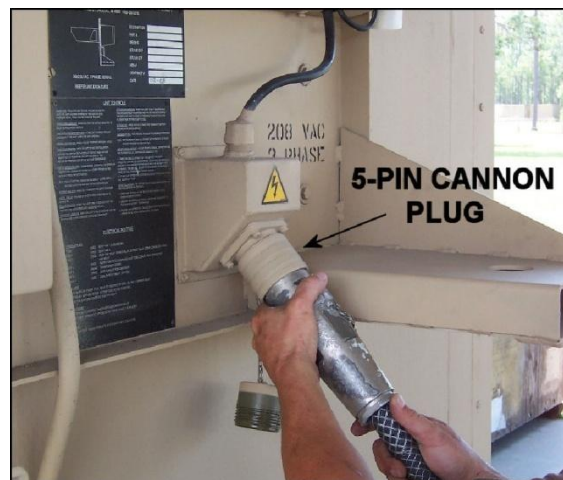
Figure 3.13. Power Supply Cable Connection to Refrigeration Unit.
