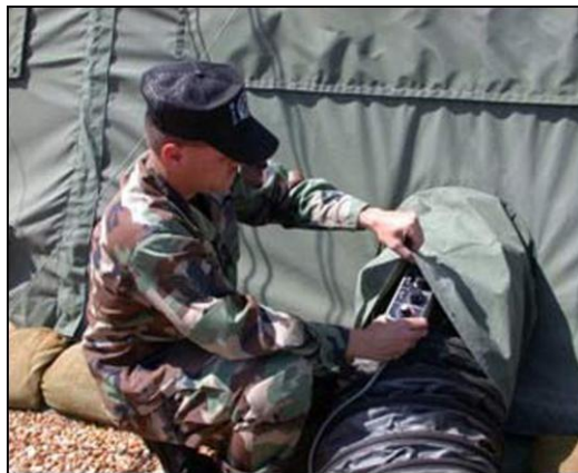
Figure 4.4. Remote Control Panel and Cable Routed Inside Shelter.
