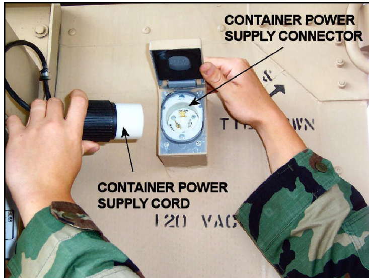
Figure 3.14. Container Power Supply Cord Connection.
