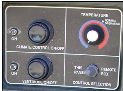
Figure 4.3. Master Control Panel.
