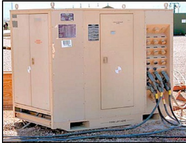
Figure 2.11. Secondary Power Cables Connected to SDC.
