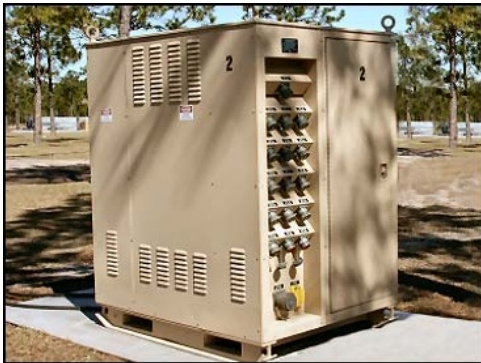
Figure 2.4. Secondary Distribution Center (SDC), Low Voltage Side.
