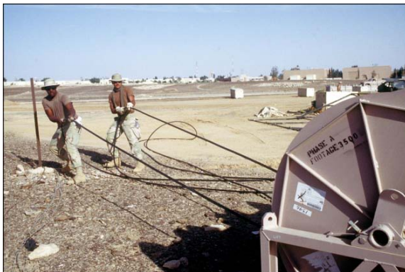
Figure 4.11. Primary Electrical Distribution Cable and Reel.
